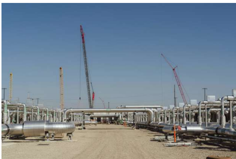
Part of the massive cooling system needed for the data center.
